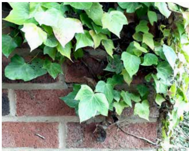
Ivy can have a serious impact on brickwork
