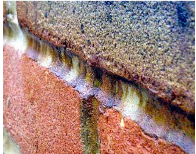
Iron staining visible on a mortar joint
