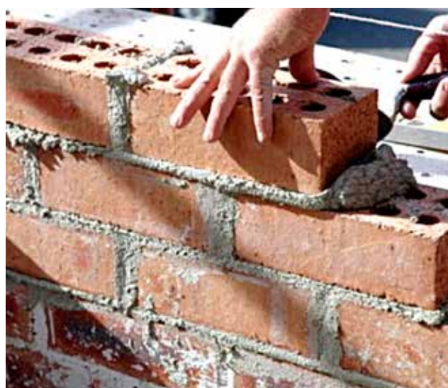
Efflorescence on brickwork under construction
