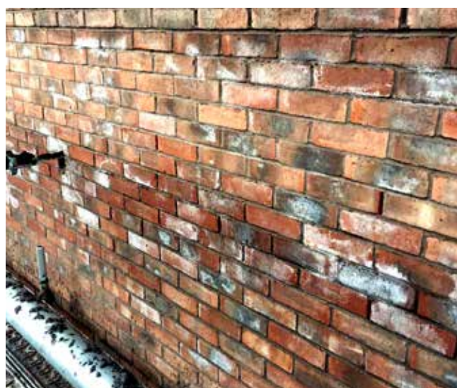
Efflorescence on brickwork under construction
