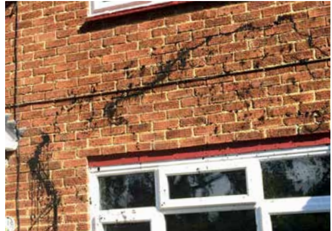
Tar stain on a textured brick
