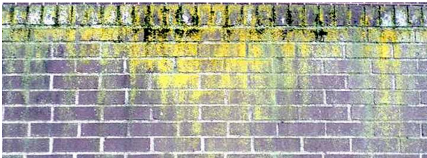
Picture framing likely due to saturation during construction
