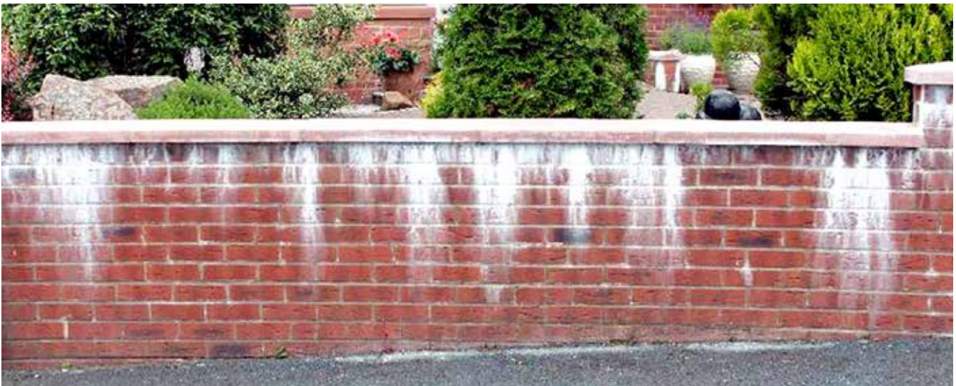
Lime staining caused by runoff from a concrete coping
