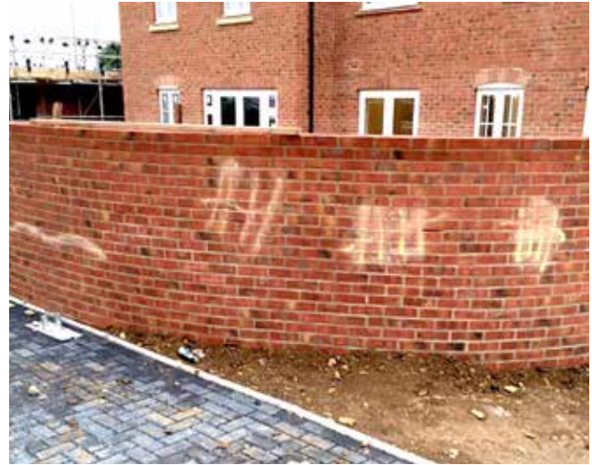
Vandalism on a building site
