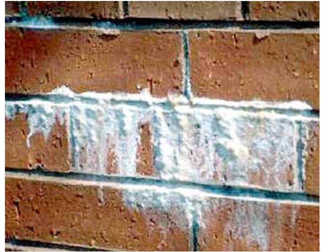
A severe case of lime staining
