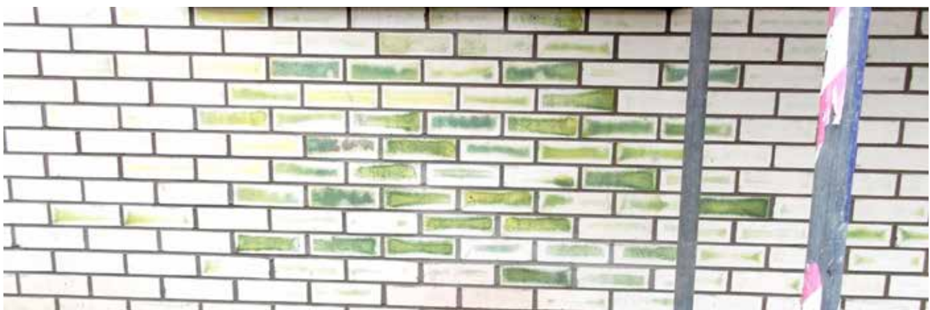
Vanadium staining visible on light brickwork
