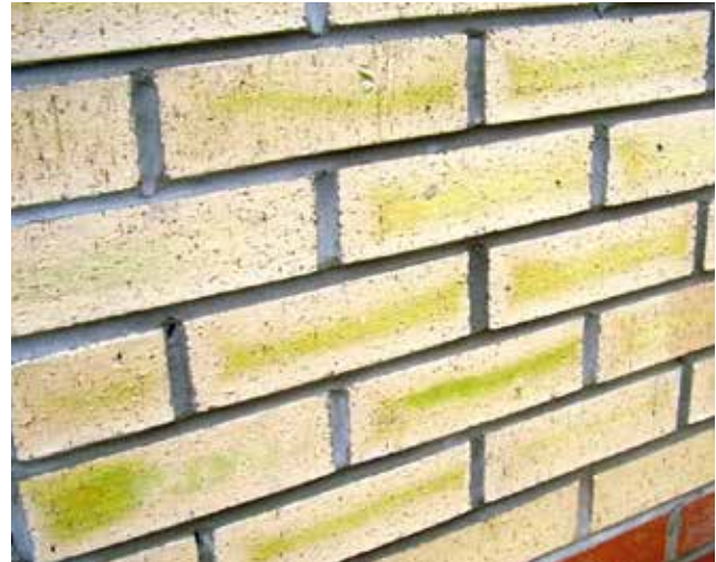
Saturation of light bricks can result in Vanadium staining
