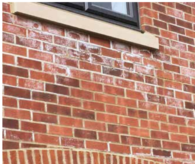
Efflorescence is the most common form of brick staining
