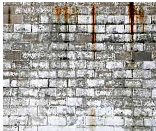
Staining from iron fixings into brickwork
