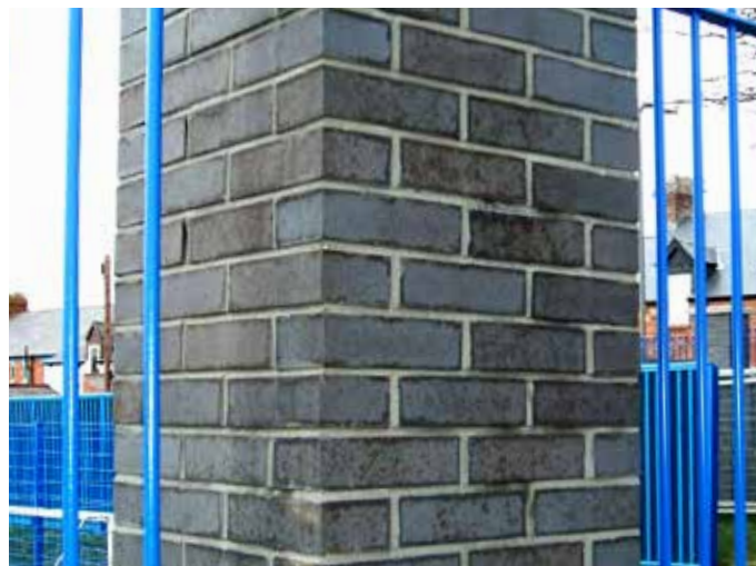
Iron staining visible on mortar joint
