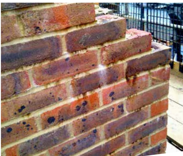
Staining on saturated brickwork
