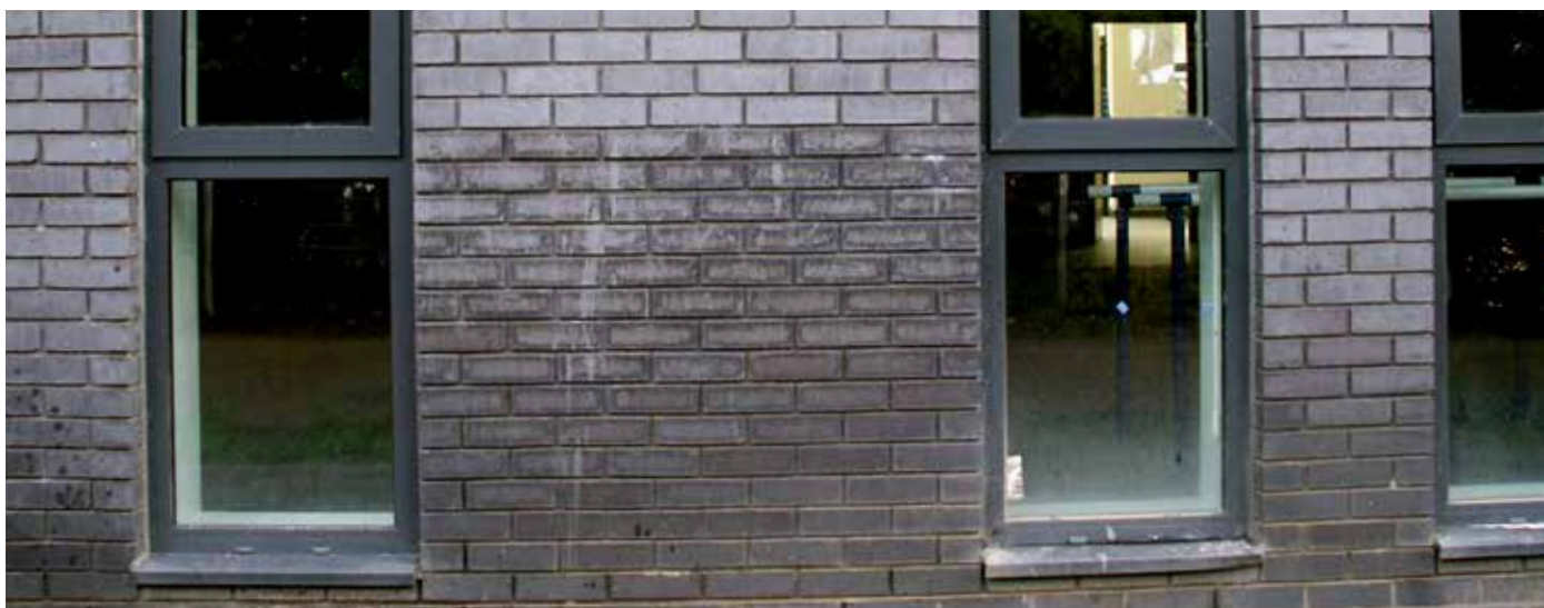
Picture framing likely due to saturation during construction
