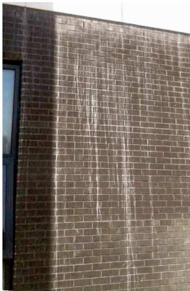
Staining from runoff over adjacent concrete
