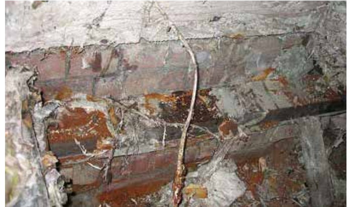
Dry rot network
