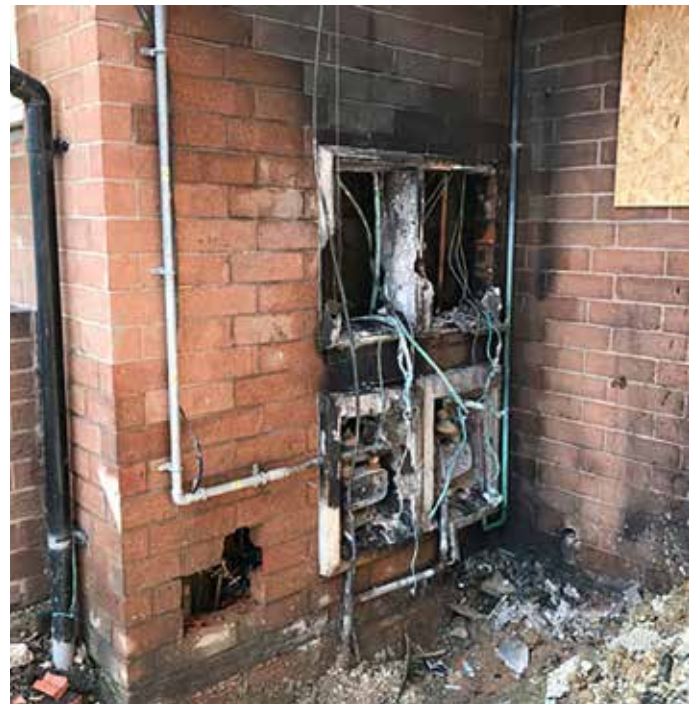
Brickwork is generally resilient to fire damage
