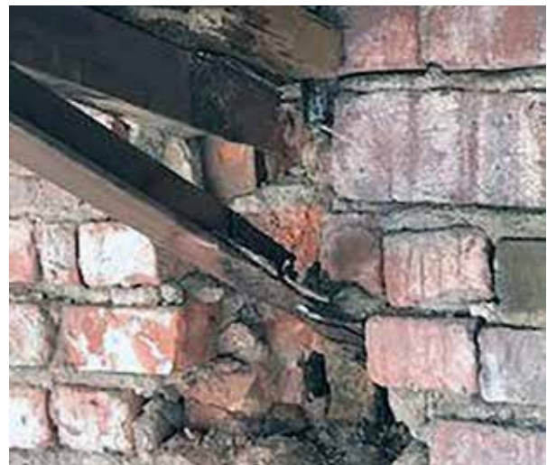
Rusting steel damaging surrounding brickwork
