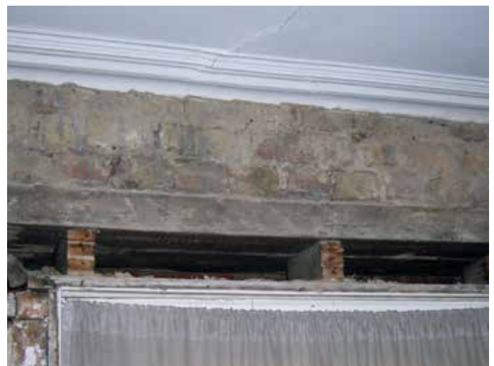
Fine crack above timber lintel
