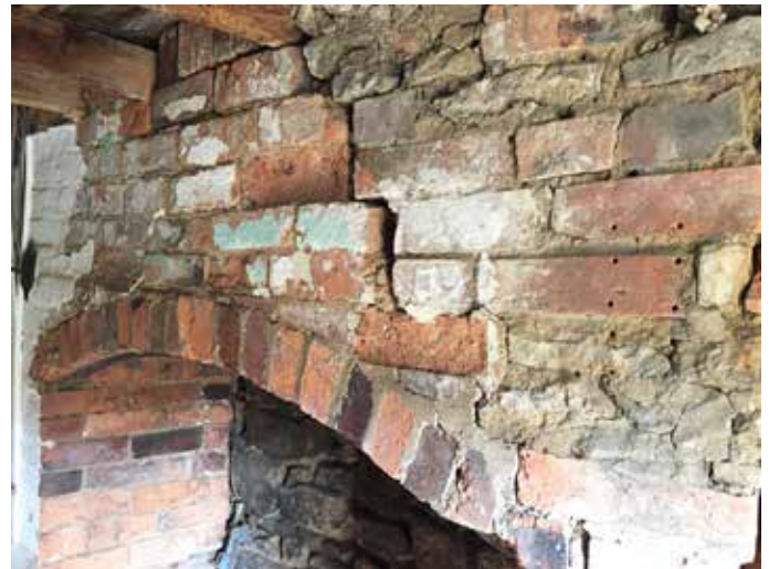
Cracked chimney breast requiring stabilisation
