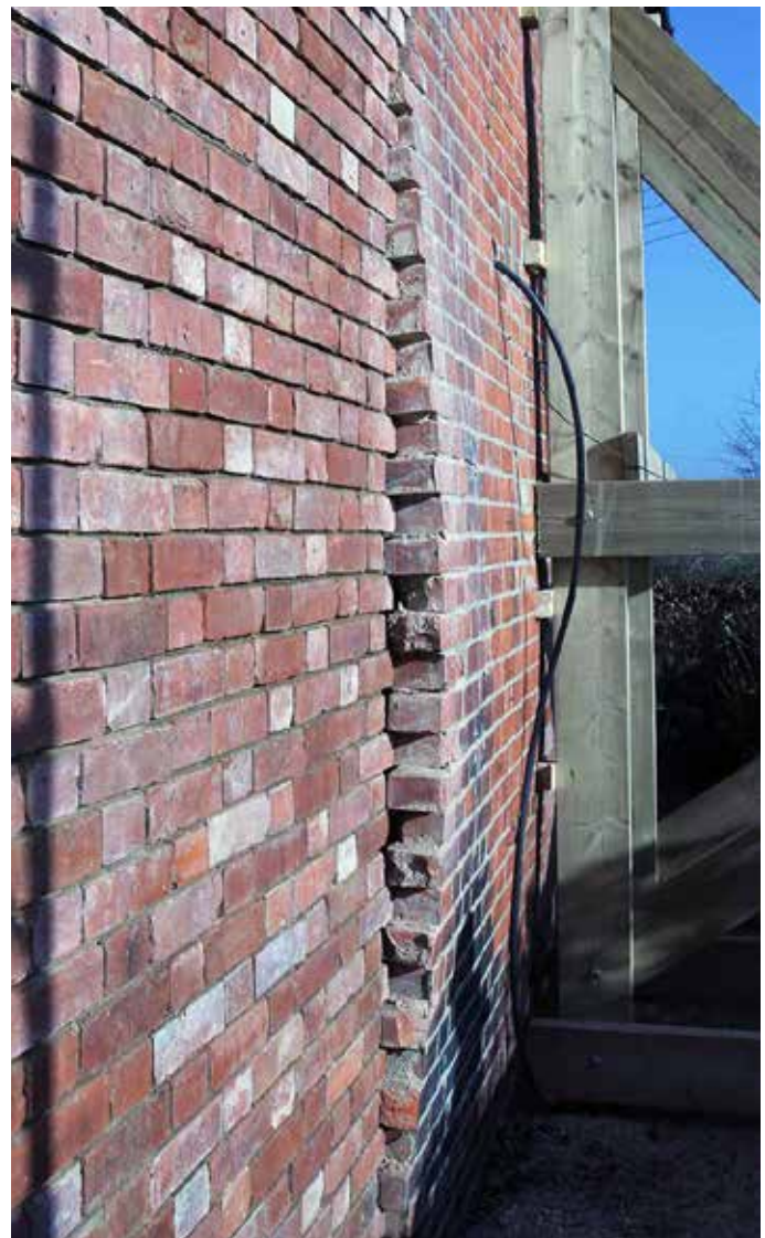
Bulging brickwork probably due to missing/failed wall ties.
