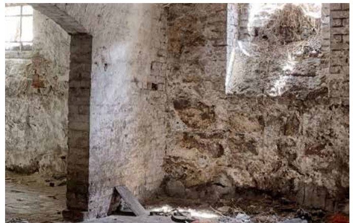
Water penetration of Brickwork
