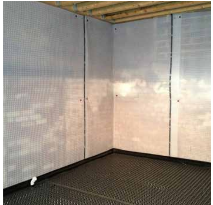
Basement floor and wall tanking membrane
