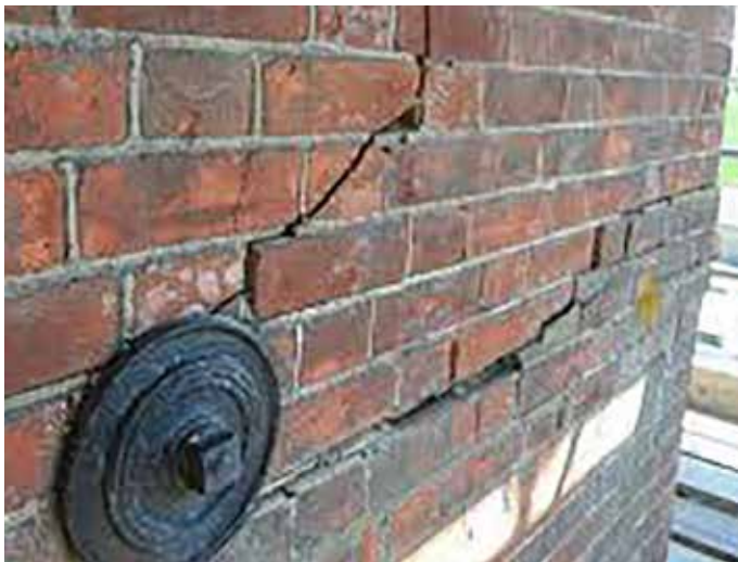
Cracking around a historic patress plate
