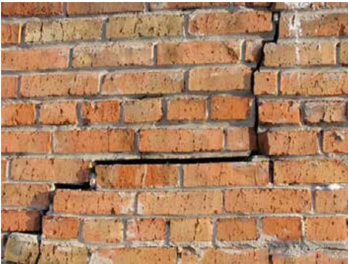
Differential settlement moving bricks down and out of plane
