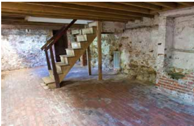
Water penetration of Brickwork
