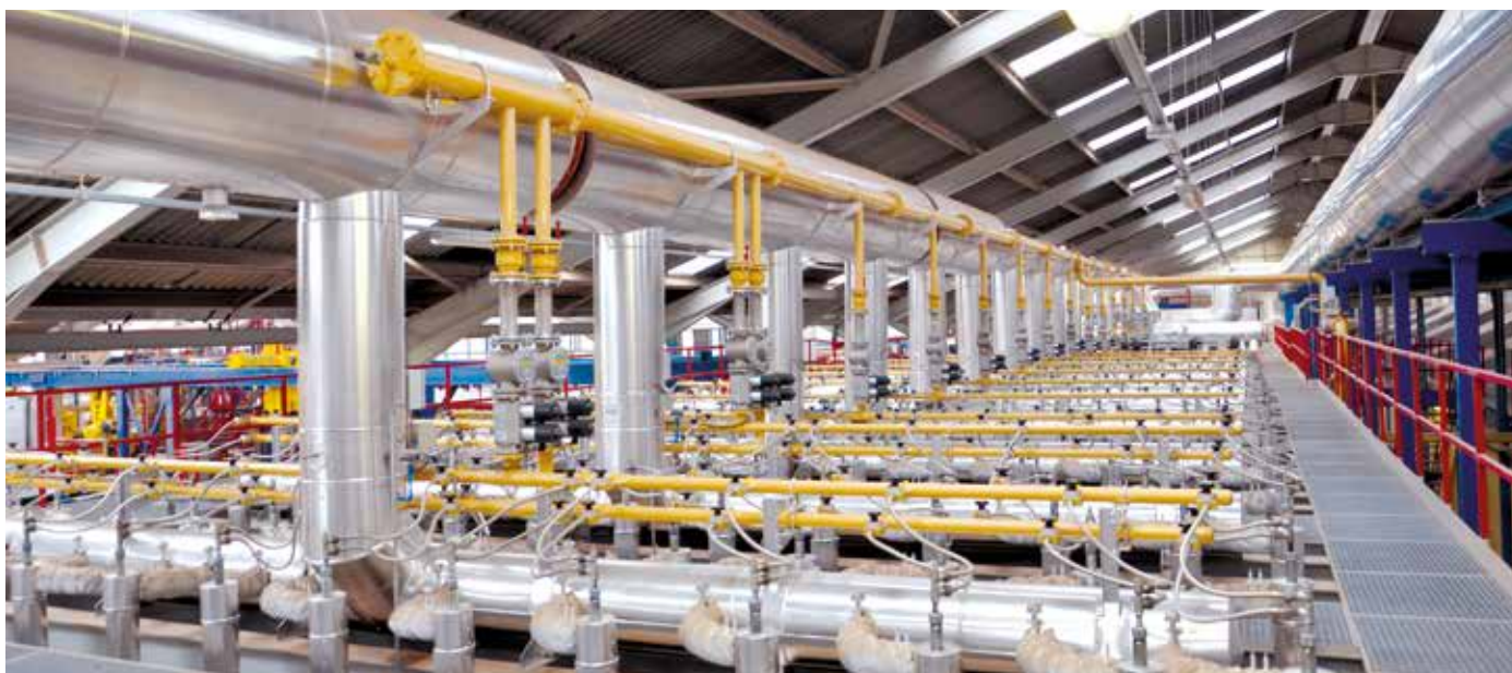
Detail of the top of a 'Tunnel Kiln'
