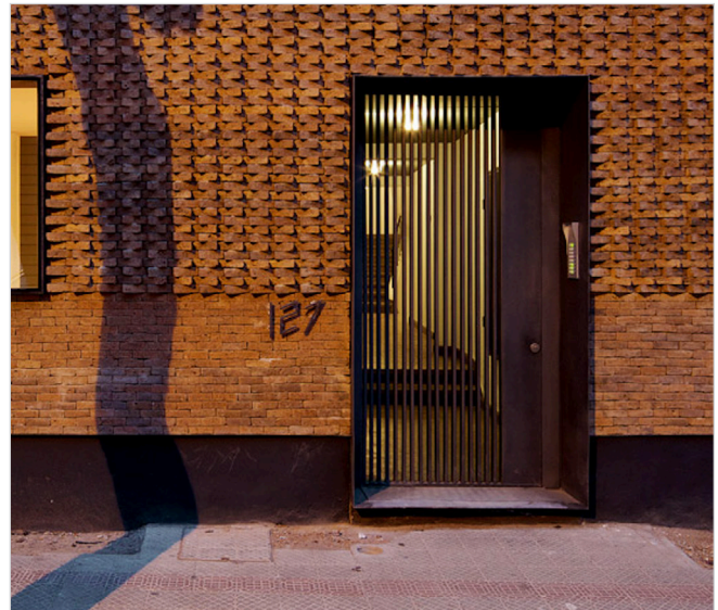
Alternate courses of stretcher bond angles at 30° from the direction of the brickwork.
