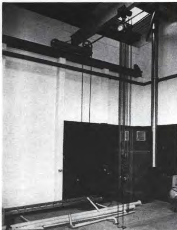
Above Detail of workshop interior, Howley Park Brickworks. Crane gantry rails are supported on 215 mm square piers bonded into the diaphragm walls at alternate rib positions. Design of brick diaphragm walls
