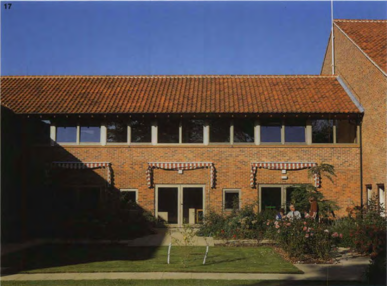
17 & 18. BUPA Hospital, Havant. The first floor link area between the wards and the operating theatres was required by the architects to be given ample natural light. To achieve this, continuous windows for the full length of the link were needed, resulting in an unrestrained cantilevering brick wall. To resist the lateral loads on this cavity wall post-tensioning was utilised, with the post-tensioning rods cast into the first floor slab and taken up the cavity of the two leaf brick wall. Architect: Lambert Scott & Innes. Consulting engineer: Curtins
